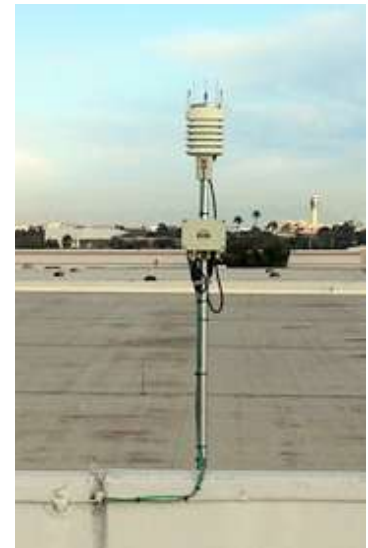
GoDaddy's Orion Weather Station installation in Arizona
